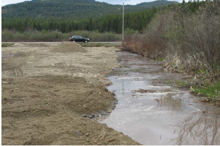
East side of the lot showing strip of excavated ground that was being filled when EPA officials arrived, taken during 2007 site visit.
