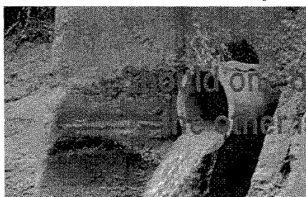
Wastewater Treatment Plant Discharge
